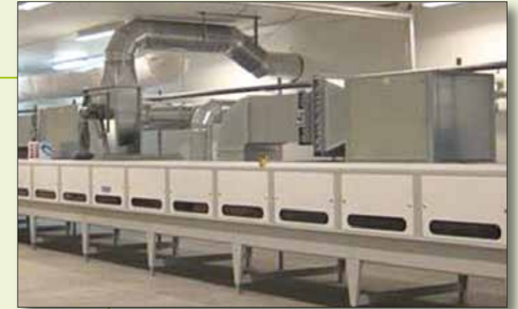
Jet drying zone with IRK lamp
